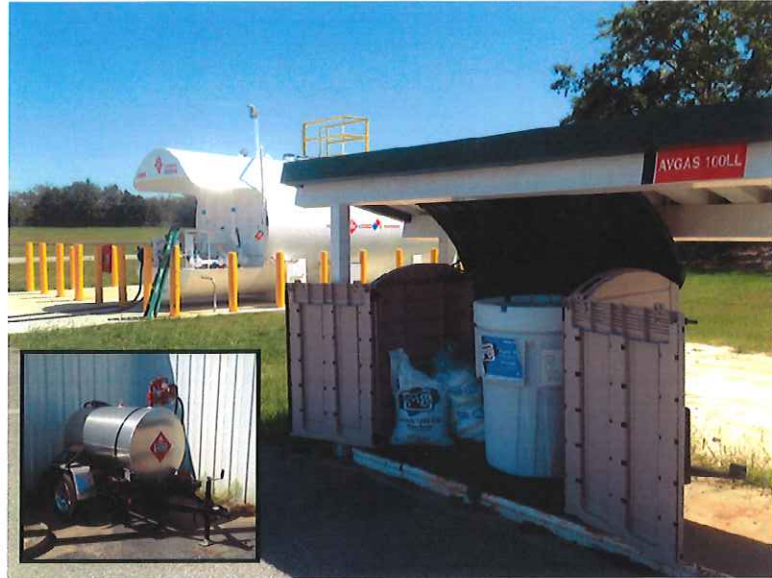
Above ground fuel tank, portable tank, and spill response kit.
