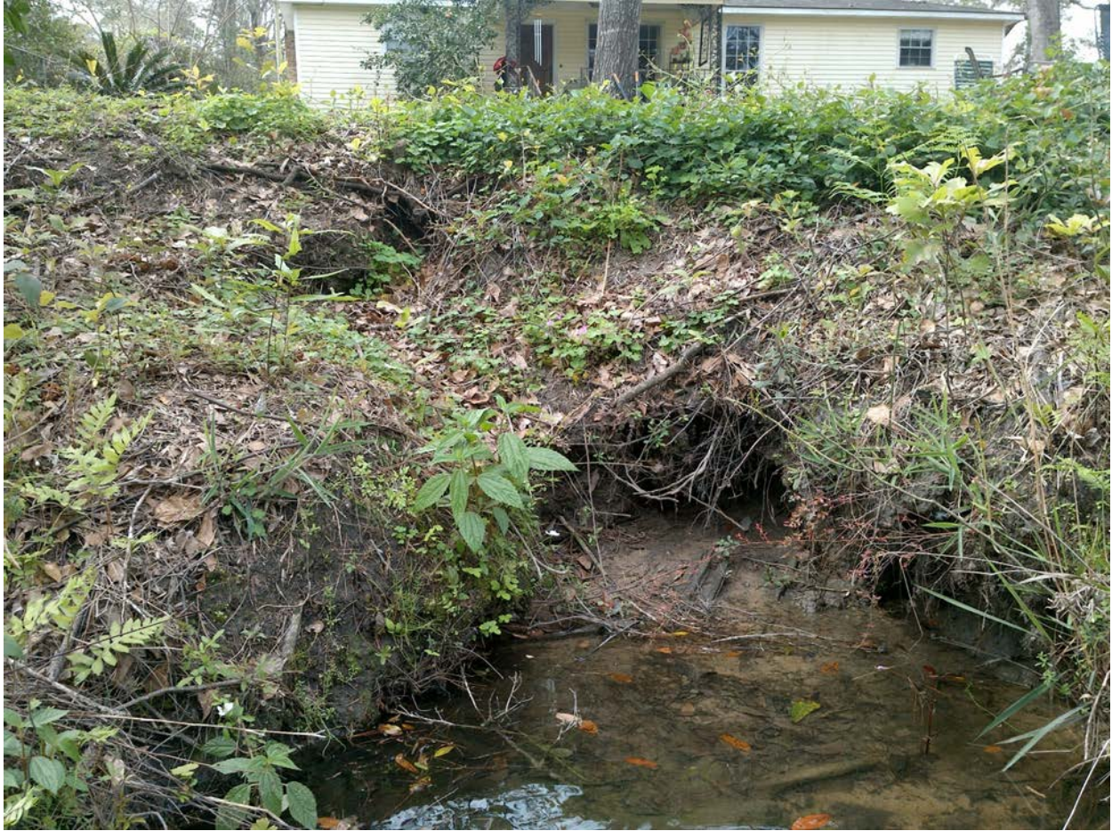
Figure 7.9 Bank Failure at Residence Along Wolf Creek
