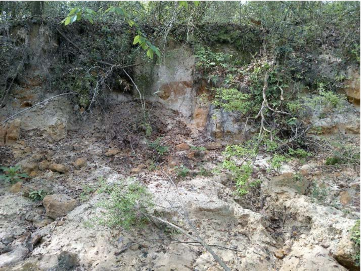
Figure 5.12 Example of Bank Instability/Sloughing Along Wolf Creek
